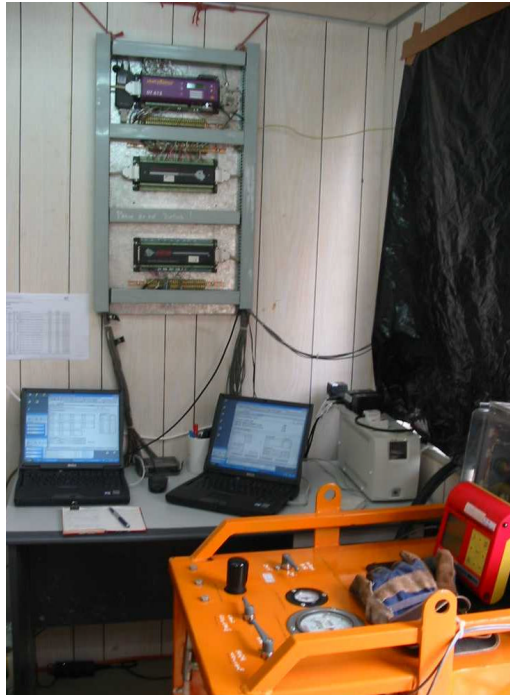
Computerised data acquisition and pile load control systems, and computer controlled pumping system
